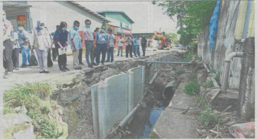
The collapsed drain along Jalan Industri 9, Kampung Baru Sungai Buloh is being repaired at a cost of RM800,000.
